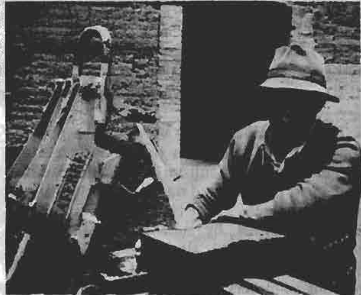
FIGURES 353 AND 354: PRODUCTION OF 5,500 BLOCKS WITH THE "CRATerre" PRESS; PEASANT COMMUNITY OF COLPAR. LOWER PHOTO: DETAIL.
