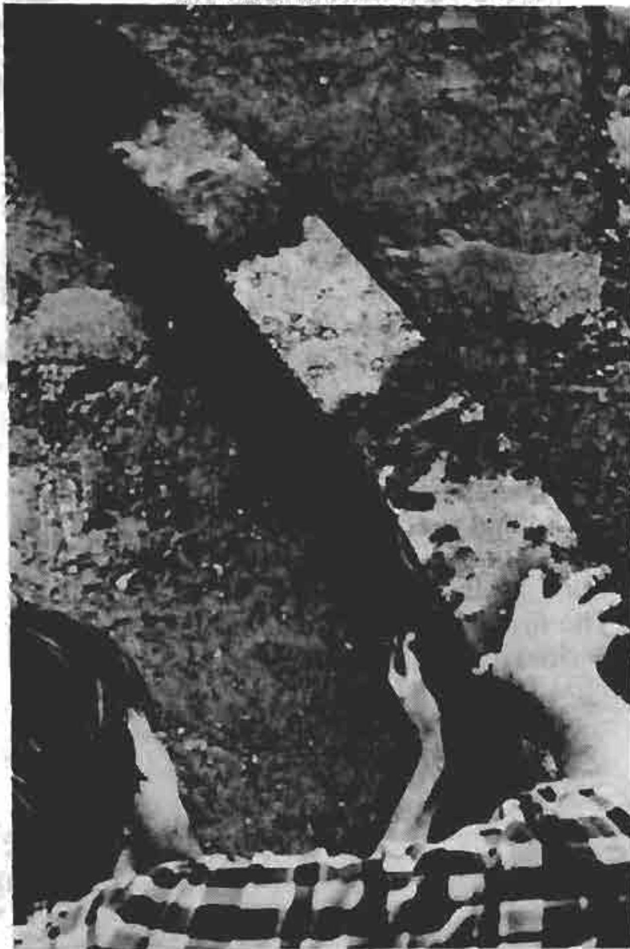
FIGURE 312: THE BRICKS ARE LAID ON EDGE: THE VAULT IS THEN 15 cm THICK.
